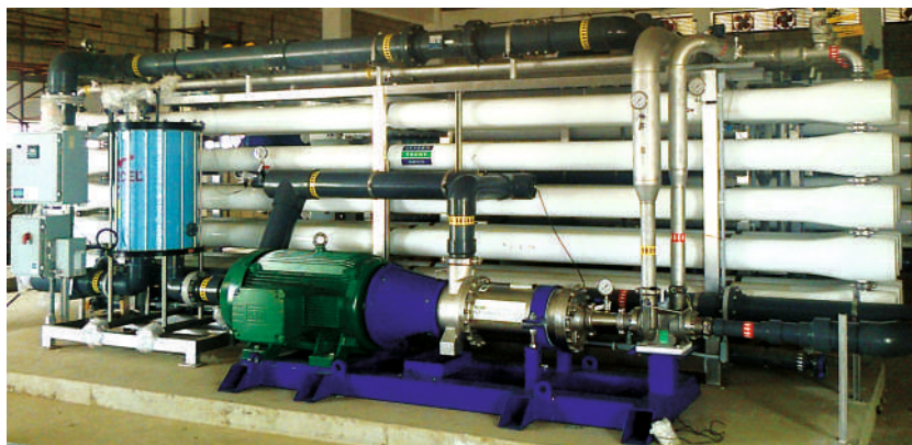
Byco Oil Refinery Seawater Desalination
