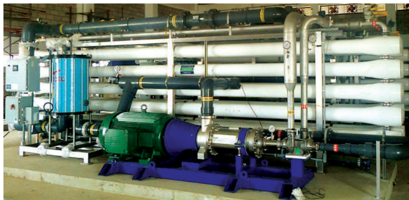
Byco Oil Refinery Seawater Desalination
